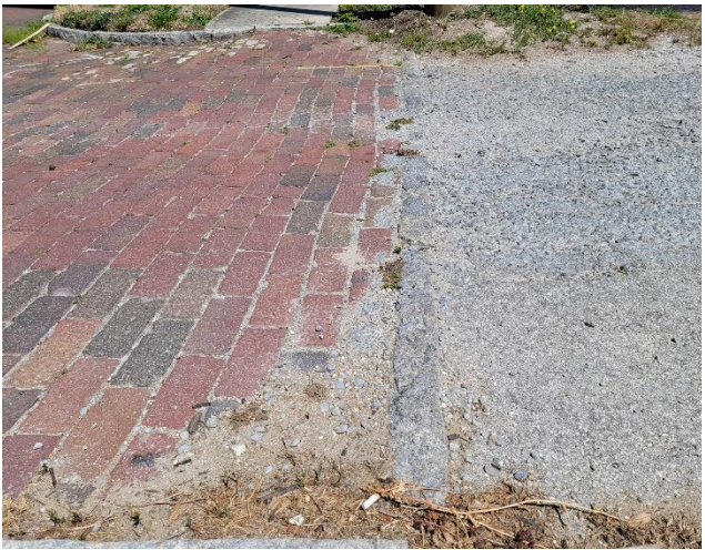
Figure 5. West end of alley looking north, showing what appears to be the end of historic brick and beginning of paving.
